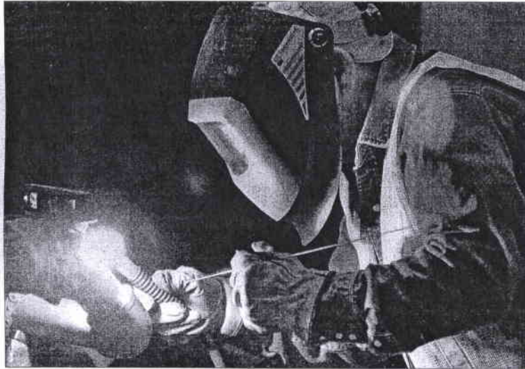
A worker welds at the dewatering facility at 1611 State St., Green Bay, in preparation for the Fox River PCB dredging project, which is scheduled to begin this week prior to the federal government's Friday deadline. H. Marc Larson/Press-Gazette
