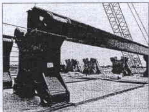
Workers install filter press frames to the Fox River Cleanup Group Green Bay Processing Facility in Green Bay.
